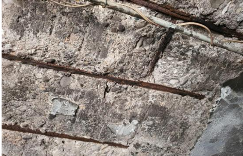
Figure 5. Corrosion in reinforce bars
