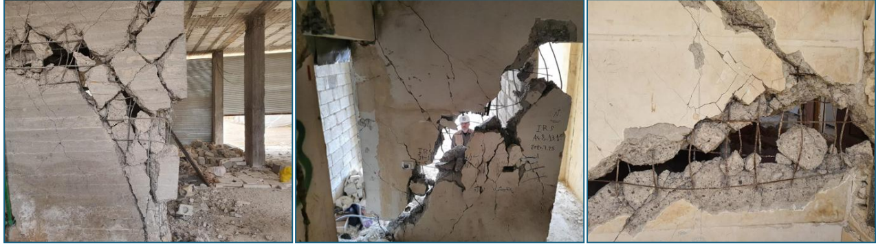
Figure 8. Observed damages in the shear walls
