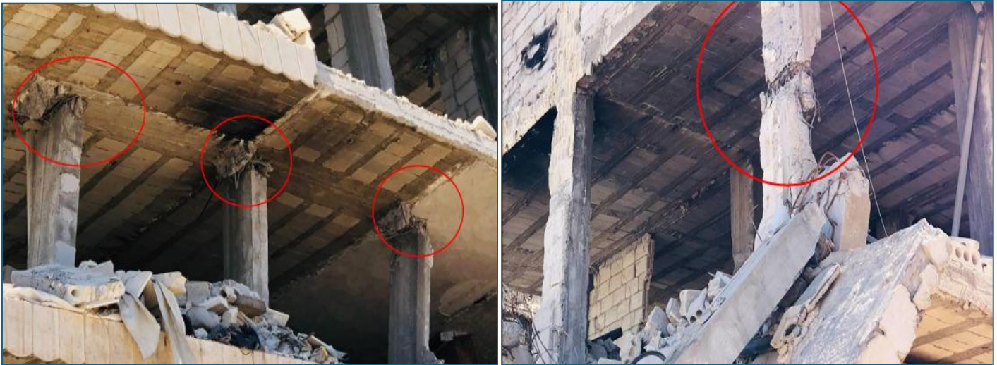
Figure 7. The insufficient cross-sections in structural elements
