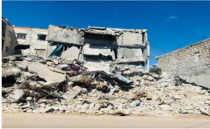
Figure 2. Totally collapsed building due to the poor concrete quality in Cinderes
