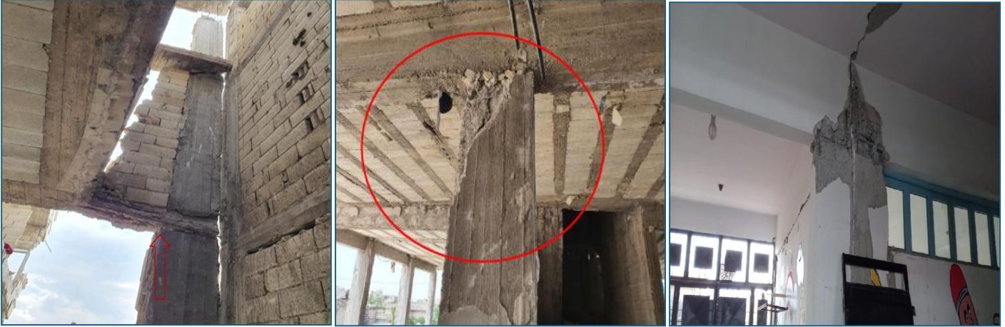
Figure 6. Plastic joint formations in columns
