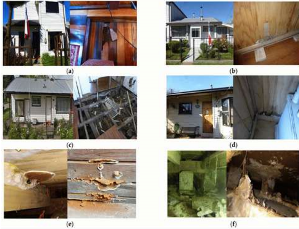
Figure 4. (a) Cracks and abrasion damages caused by moisture in wood, (b) fungi that form due to high relative moisture content in wood, (c) deterioration in wooden flooring caused by capillary water absorption, (d) cracks and abrasion damage caused by moisture on wooden walls, (e) wooden flooring and rot under the outer covering, (f) biological deterioration caused by moisture under the wooden floor (Espinoza Maldonado et al., 2024)
