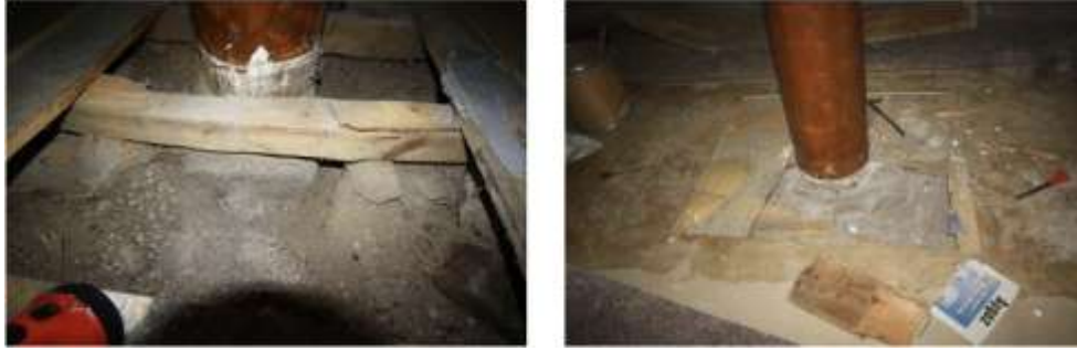
Figure 12. Harim northeast direction middle strut pedestal and Harim southeast direction middle strut pedestal
