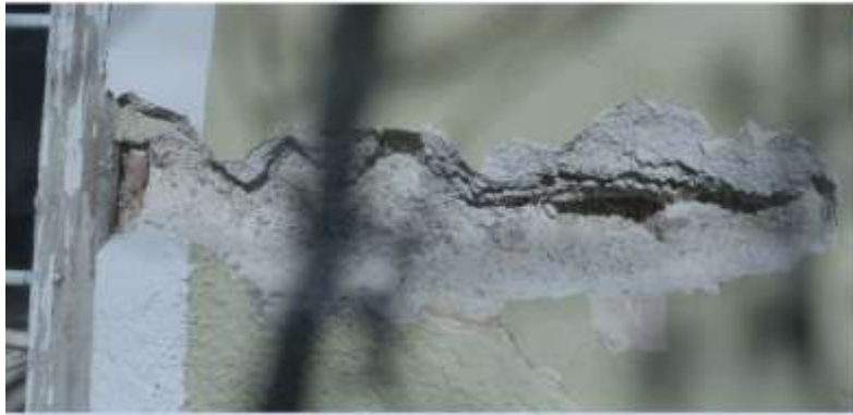
Figure 10. Rubble stone masonry revealed at the end of the plaster scraping of the southwest wall of the harim
