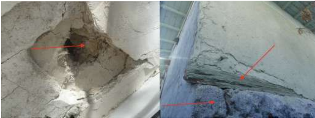
Figure 14. The result of plaster scraping on the upper part of the southwest window of the Harim and the wooden beams and rubble stone masonry on the northeast façade of the Harim
