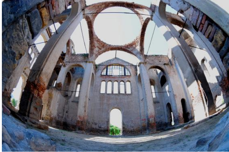
Figure 7. Deformations in masonry pillar ( https://www.osmaneli.bel.tr/hagios-georgios-kilisesi )
