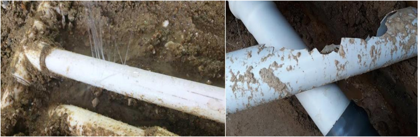
Figure 1. Water loss due to cracks in water pipes
